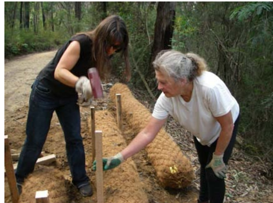
Above: Dori Leadle (Hazelbrook Streamwatch volunteer) and Anne Carey install coir logs to prevent sedimentation of a Bedford Creek tributary
